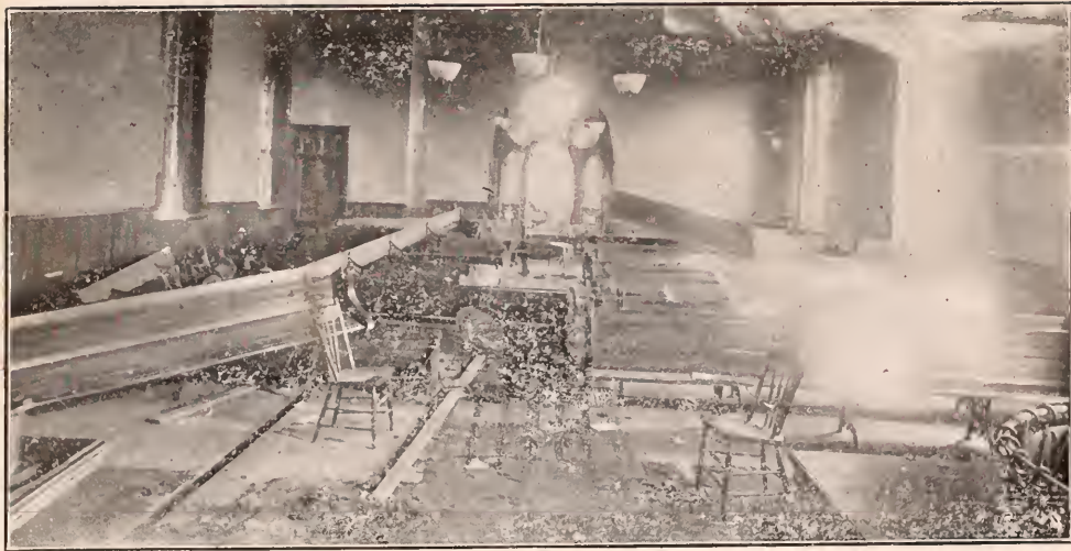
Church of God, Washingtonboro, Pa., wrecked by Acetylene Gas Plant explosion, 7.55 p. m. 3-19-'07.
